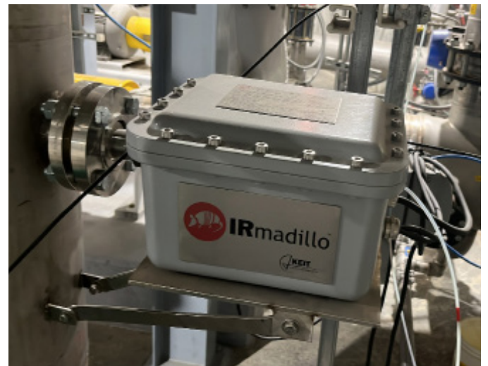
Image: IRmadillo spectrometer mounted in the recirculation loop of an ethanol fermenter
